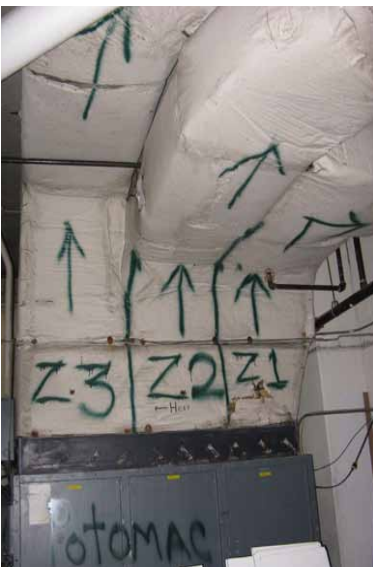
Auditors inventory and measure equipment efficiency.
